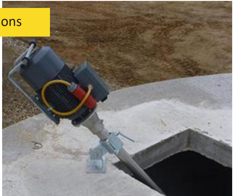
Mounted in reception tank
